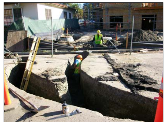
Below: The “less glamorous” work of construction is trenching for the new water system! These utility workers fit pipes and do remarkable work in very narrow passages.
