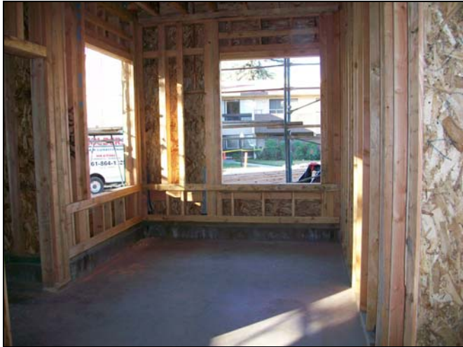
Left: A view of the interior framing of the Norton Garden Building. Electrical and plumbing work is in process simultaneous with the framing. At this point in the process, it is possible to distinguish hallways, rooms, and views from each window.
