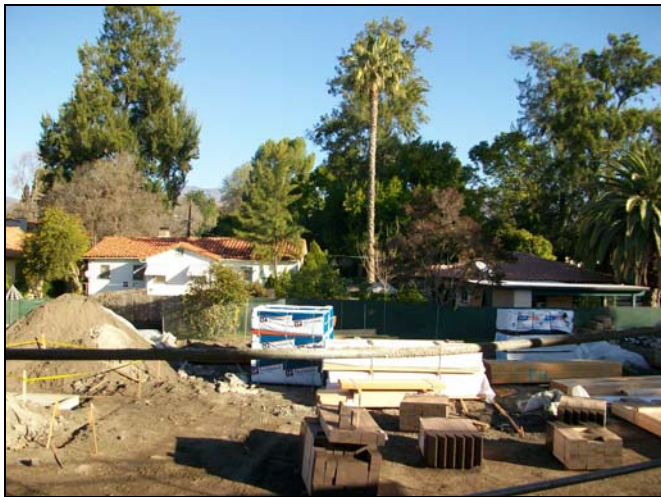
Left: Norton Garden Apartments facing north have lovely views of treetops and the mountains in the distance. Building supplies now stand in the location of the future carports.
